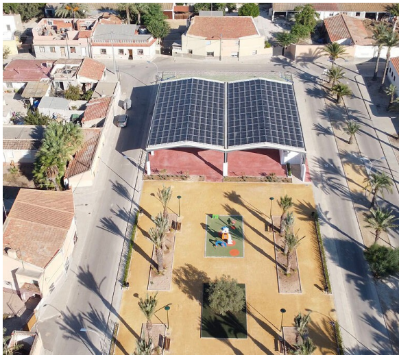
COMPTEM PHOTOVOLTAIC INSTALLATION. QUELLE: GRUPO ENERCOOP
